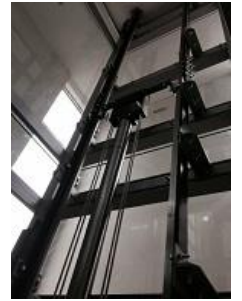
CUSTOM PAINTED MECHANICAL
